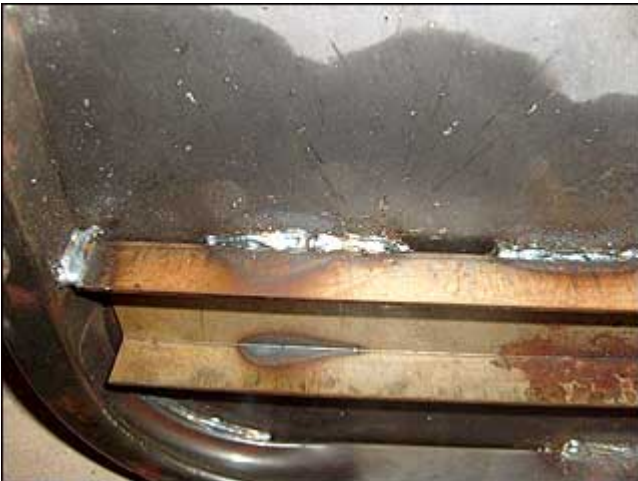
Weldings are strong but they do not have not a smooth aspect.
