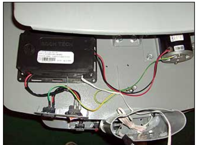
Connections are clean and all made with plugs.
